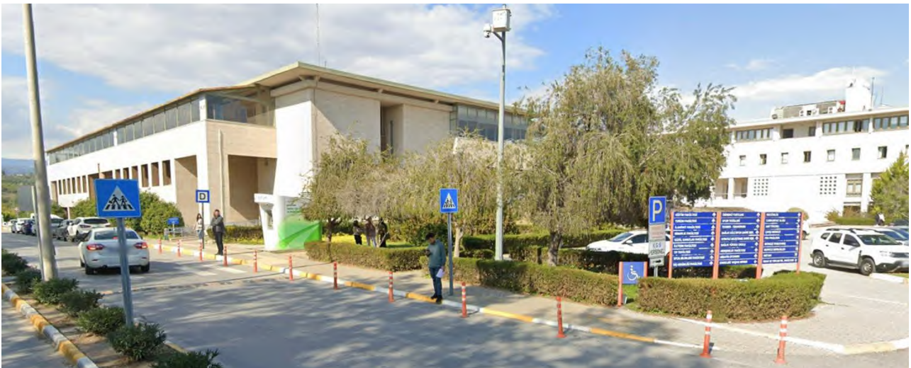
Outdoor security camera (CCTV)
