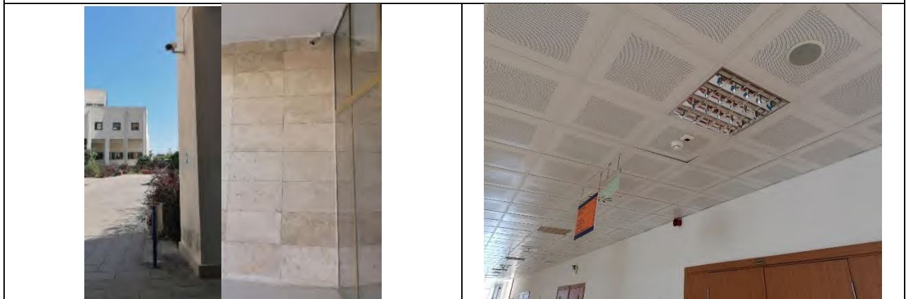
Cameras, fire sensors,
