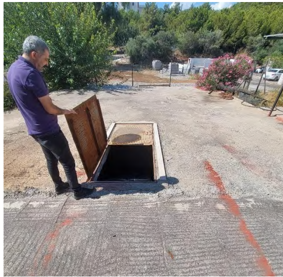
Rainwater Harvesting System - Cistern (water reservoir)
